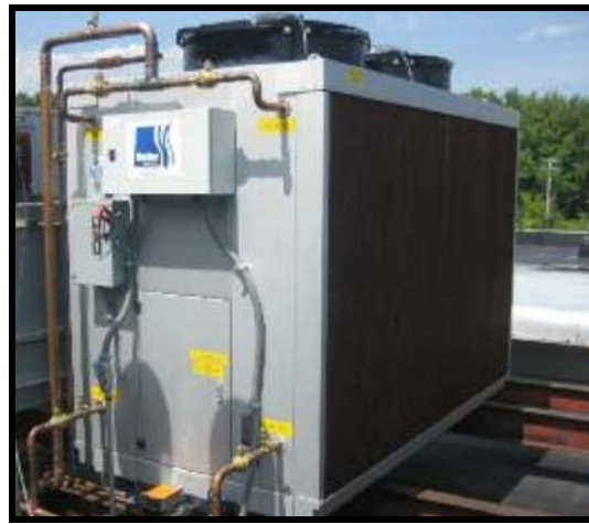
Muller 3C Hybrid Condenser mounted on structural steel.
